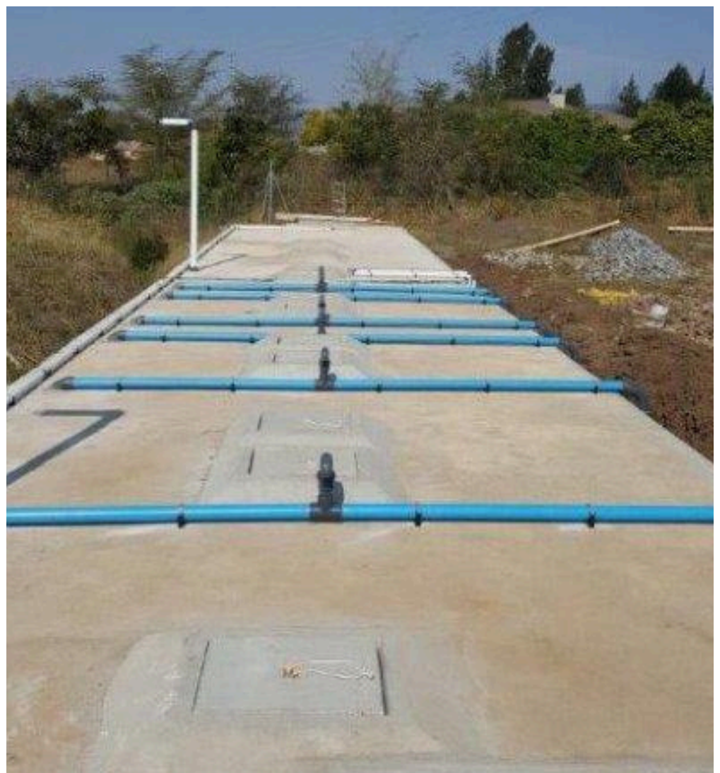
135kl concrete effluent treatment plant -Swaziland
